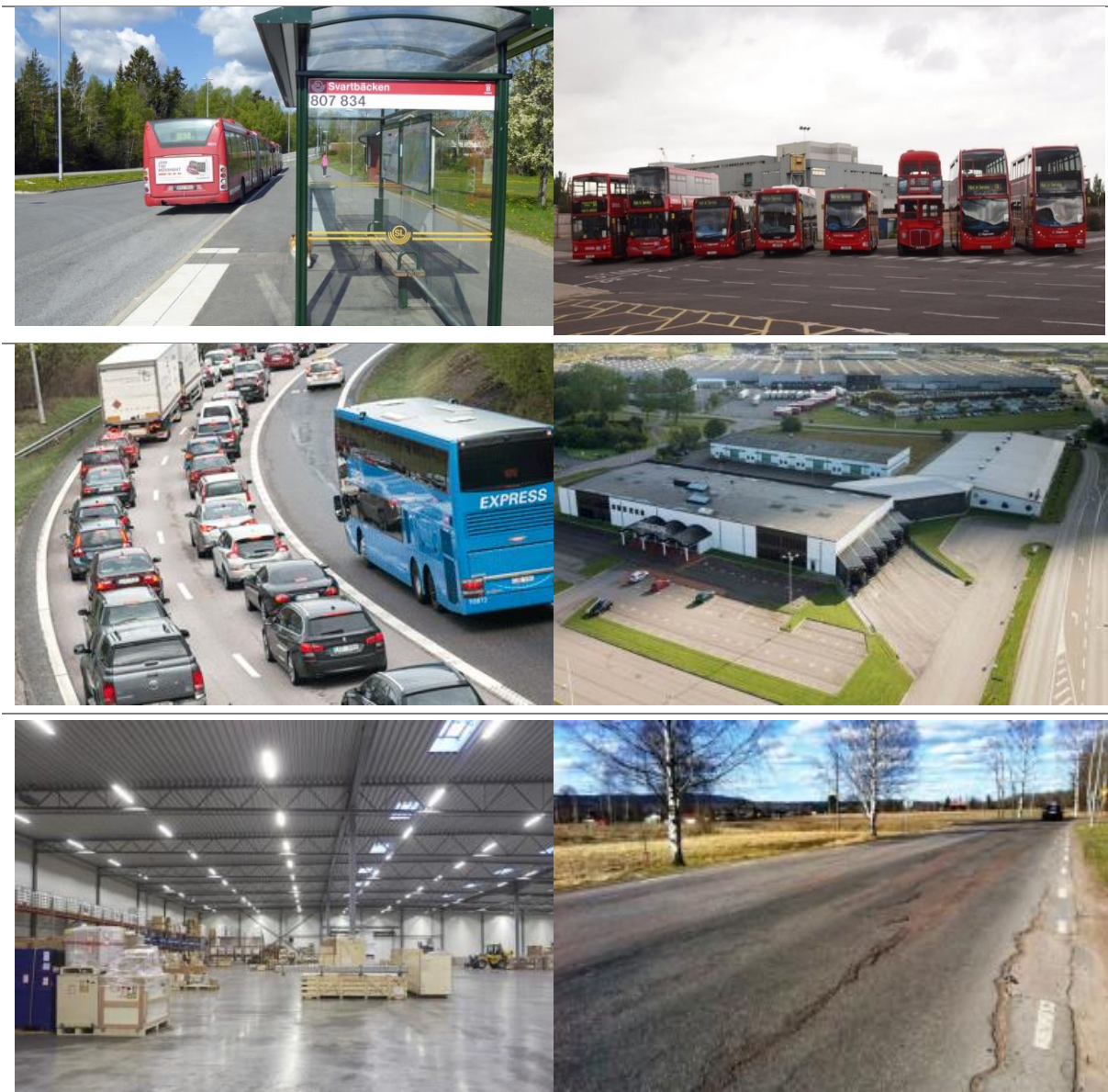
Figure 1 Examples of asphalt pavement distresses in bus stops, stations and paths, logistic and warehouse areas and high-weight trafficked roads
